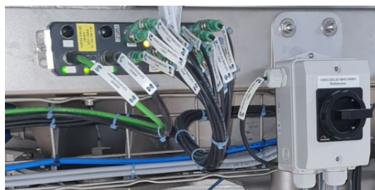
Decentralised I/O device IP67 (Phoenix Axioline E)
