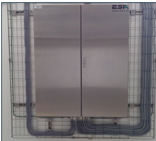
Control distributor with ET200SP modules
